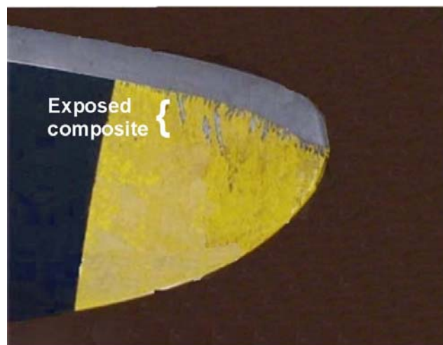
FIGURE 2-6. Composite Blade Erosion
