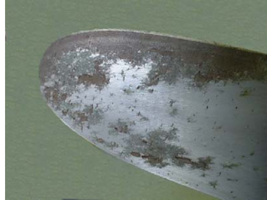
FIGURE 1-2. Polished Blade Surface Corrosion
